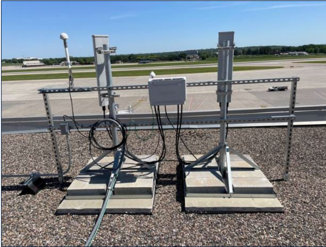
Figure 8 Nokia MBO and antenna mounted on the roof of Terminal 1
